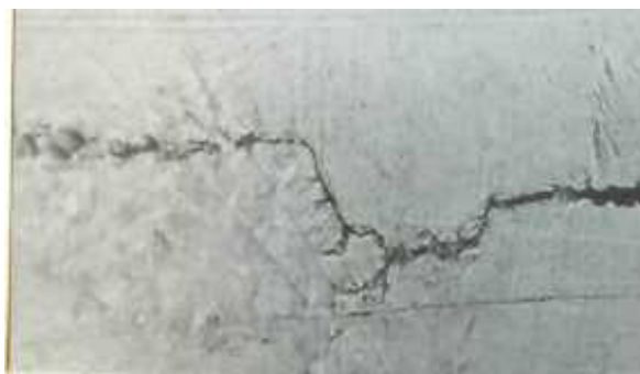
Figure 3. Formation of a new fatigue crack one of the branches
