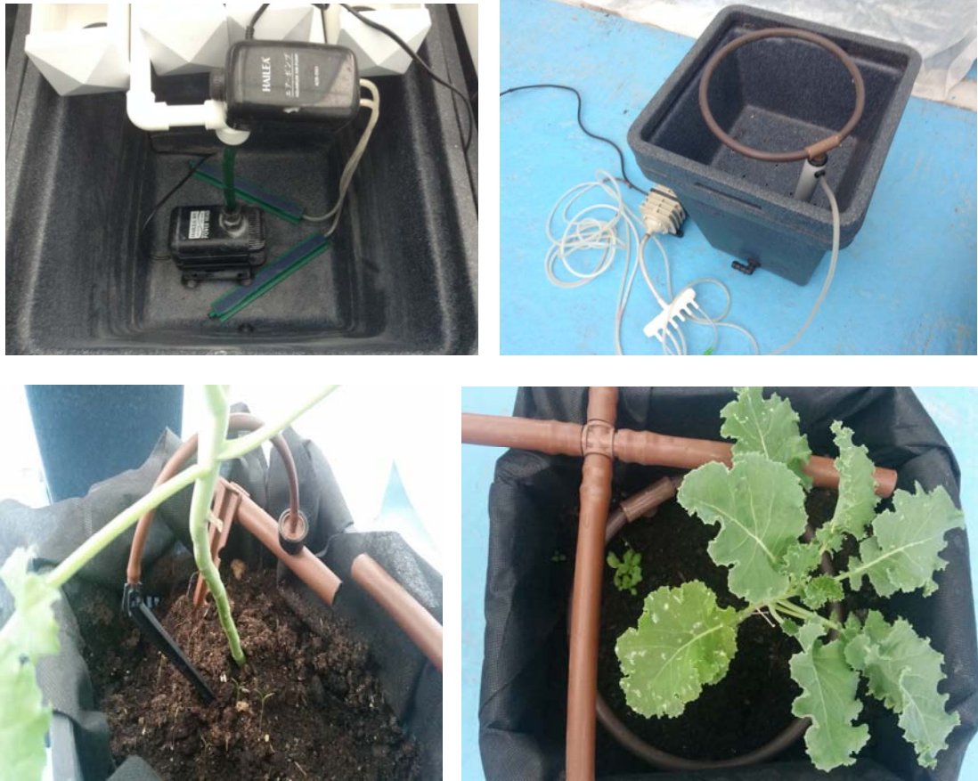
Photo 2 - Tank, water, and nutrient solution supply pump, as well as a drip irrigation system
