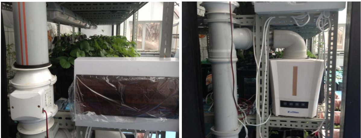
Photo 3 - Gas regulation fan (photo on the left). "Cold steam" and air ionization device and (right)
